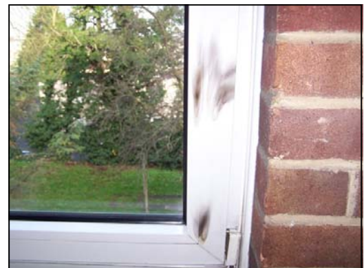
Damage caused to windows
