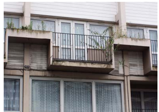
Weeds growing on balconies
