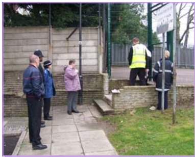
Cllr Fitzgerald and Safer Neighbourhoods Officers inspect the damaged gate
