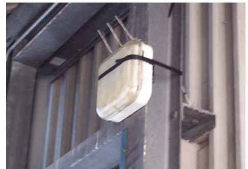
A vandalised light
