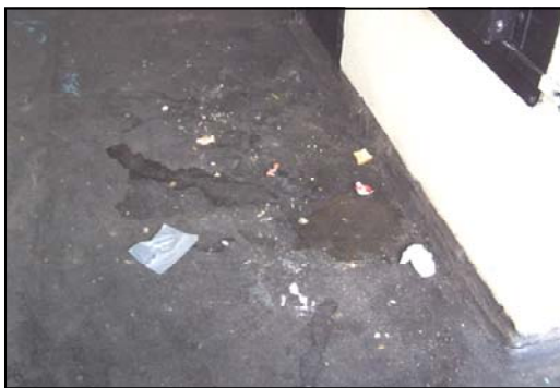
Rubbish outside a bin chute
